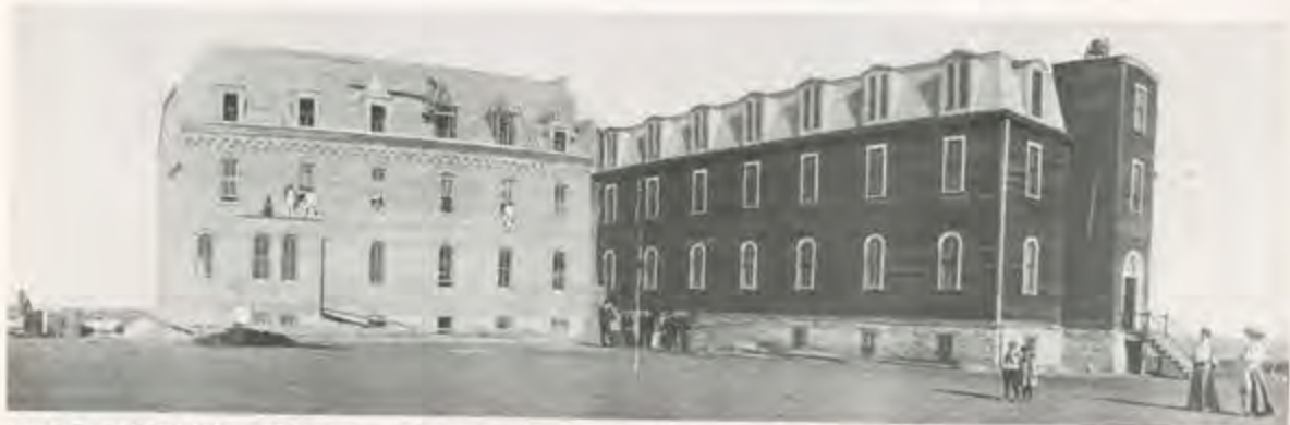
Abbot Vincent Wehrle's dream of a monastery at Richardton takes shape here as construction proceeds on the first brick section of St. Mary's Abbey in 1904. Notice the ladies from the town and a few gentlemen "inspectors" at the center of this photo as workmen are seen near, on top of, hanging from and looking out of this building which is part of the north wing of the present day Abbey quadrangle.
